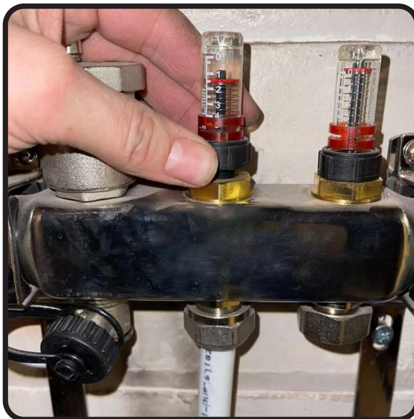
Flow meter open (collar removed)
